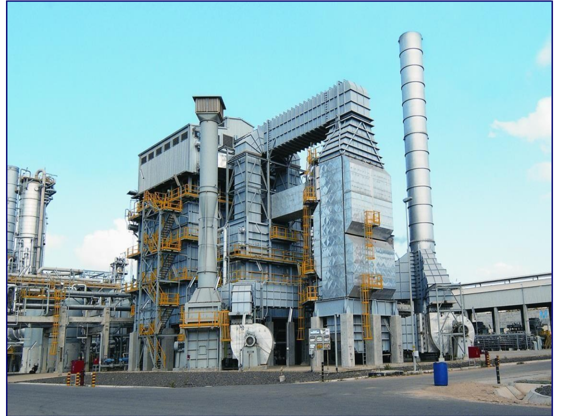
Top Fired steam reforming (Courtesy of KT Spa)
